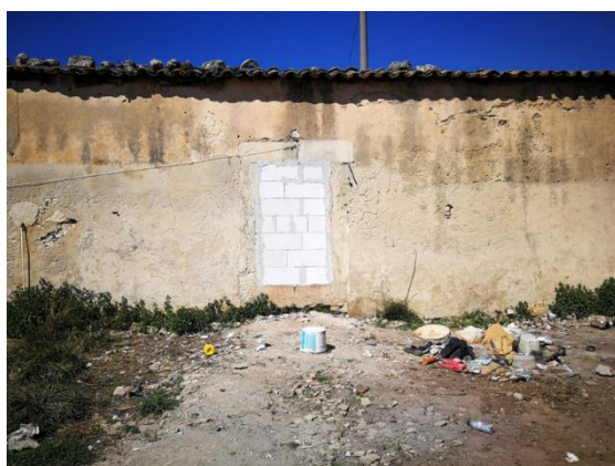
Walled-up window of the evacuated accommodation; photo Borderline Sicilia
